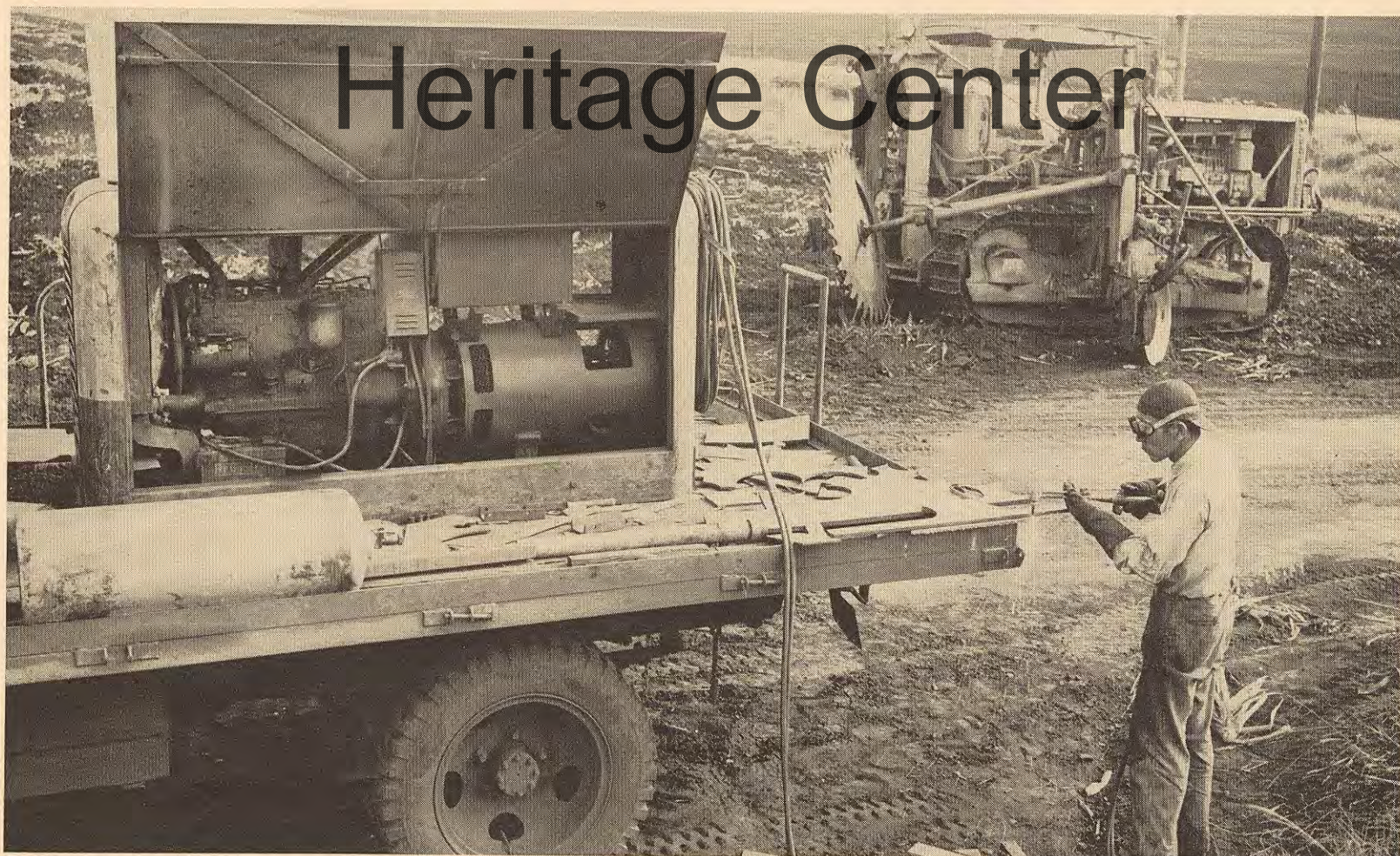
FIELD WELDING UNIT at Wahiawa. Shosaku Kimura, Leading Maint. Constr. Mech., Engineering Dept., is shown here using a cutting torch to prepare a piece of steel for use on the plantation's experimental trash sweep plow. This unit carries equipment to repair machinery in the field which otherwise would have to be taken into the shop.
